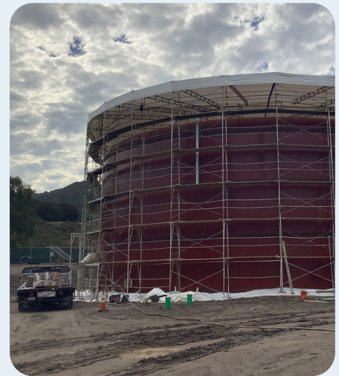
Kelt Reservoir & Pipeline (Orcutt Water System)
