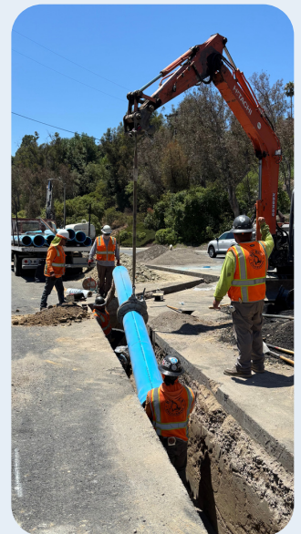
Ambervale Secondary Feeder Line
