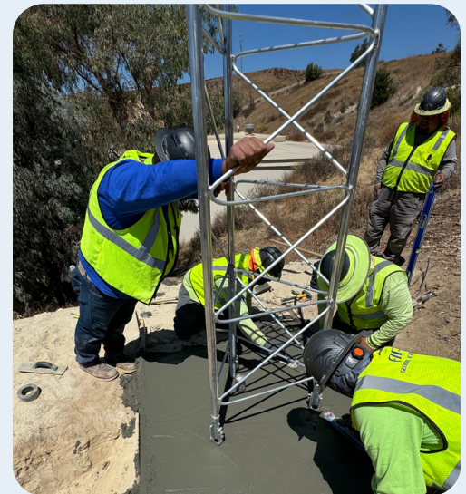
Simi Valley SCADA Upgrade
