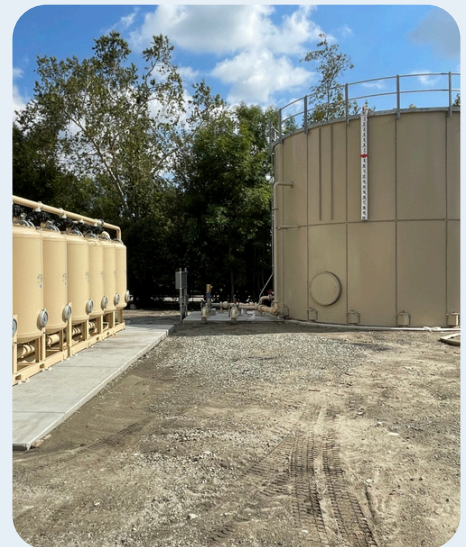
Del Monte Treatment and Booster Station
