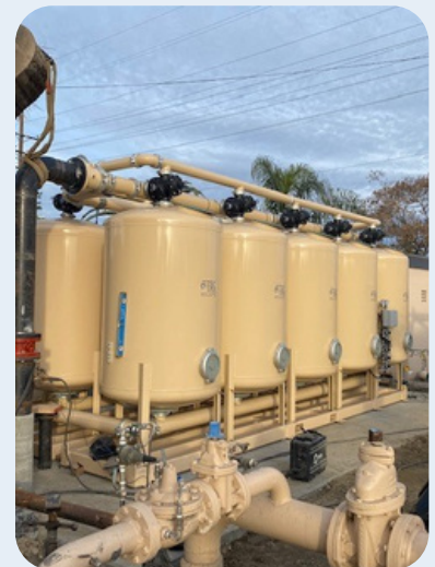
Ball Well No. 1, Iron & Manganese Removal System
