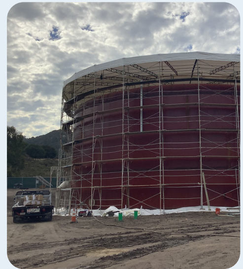
Kelt Reservoir & Pipeline (Orcutt Water System)
