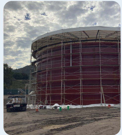
Kelt Reservoir & Pipeline (Orcutt Water System)
