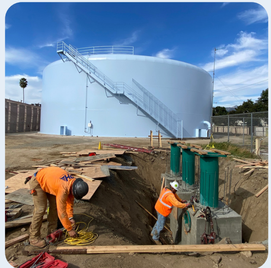
Jeffries Plant 1.25-Million-Gallon Reservoir and Booster Station
