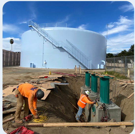
Jeffries Plant 1.25-Million-Gallon Reservoir and Booster Station
