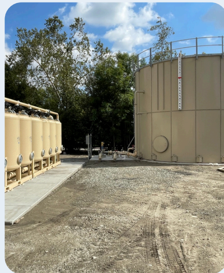
Del Monte Treatment and Booster Station
