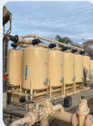
Ball Well No. 1, Iron & Manganese Removal System
