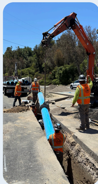
Ambervale Secondary Feeder Line
